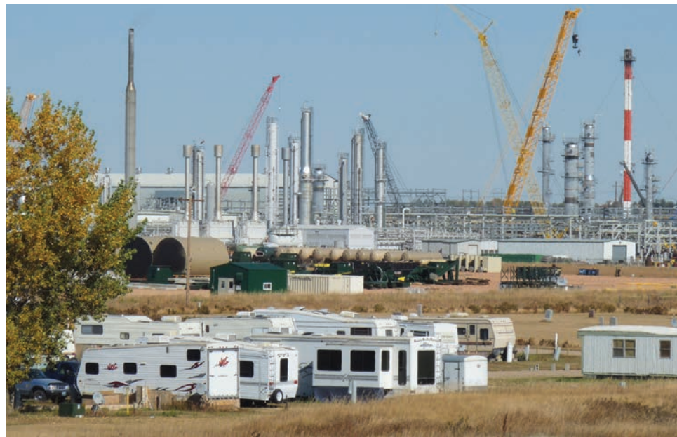
Hess is expanding and upgrading its gas processing plant in Tioga, N.D.
